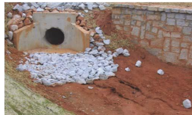
Inadequate stone coverage. Stone does not completely surround outlet pipe or prevent additional erosion from occurring.
