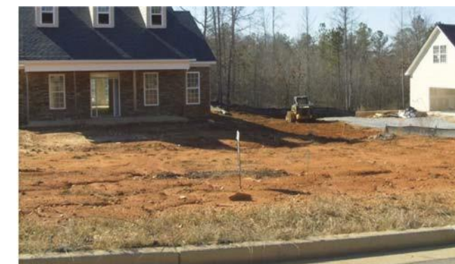
Poor vegetative cover, large bare spots (unrelated to rain events or original site conditions). Extensive erosion taking place.
