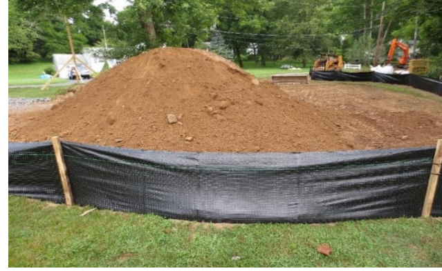
Excellent silt fence installation. Trenched in and held up using wooden stakes.
