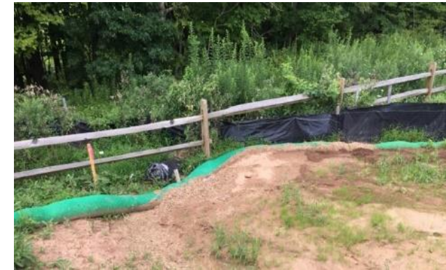
Improper installation. Fence not properly trenched, allowing sediment to pass underneath unimpeded
