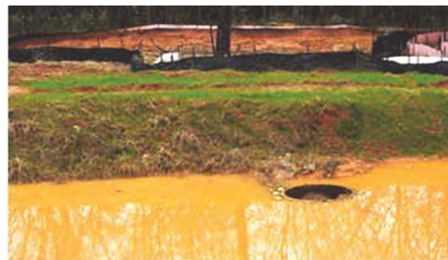
Inadequate maintenance has caused sediment basin to fill and overwhelm riser (not related to significant rain event).
