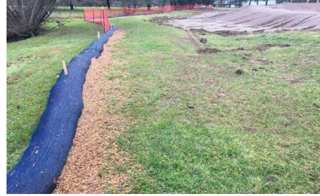
Excellent compost filter sock. Placed downhill, no torn seams or sediment build up.
