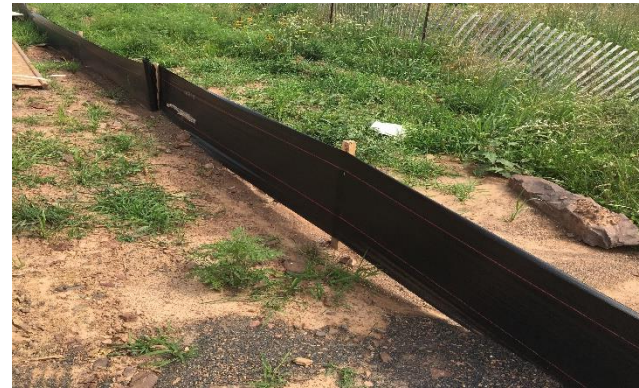
Silt fence not properly trenched when installed.
