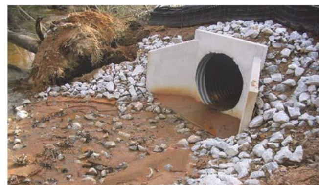
Completely inadequate stone coverage. Erosion problems occurring.
