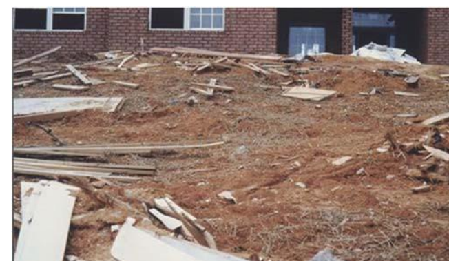
Completely inadequate coverage over a period ~2 weeks of inactivity.
