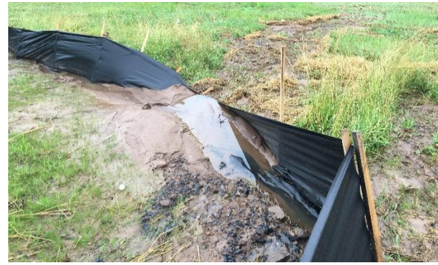
Silt fence blown out by stormwater flow and sediment. Needs to be repaired.
