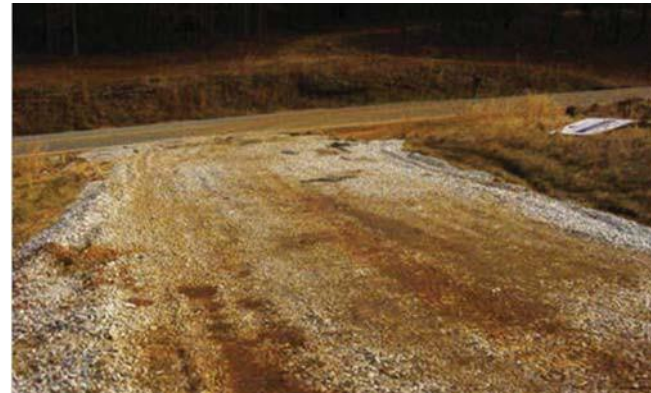
Stones are too small and coverage is inadequate. Also lacking geotextile underliner. Dirt is being tracked onto roadway.
