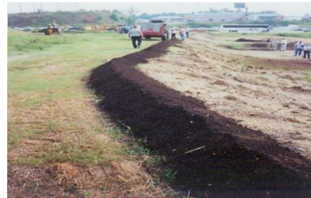
Compost filter berm. Used for sheet-flow runoff, not channelized. Could also be vegetative berm. Photo: PADEP
