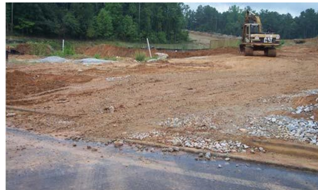
Inadequate maintenance of construction exit. Sediment and rock entering roadway.
