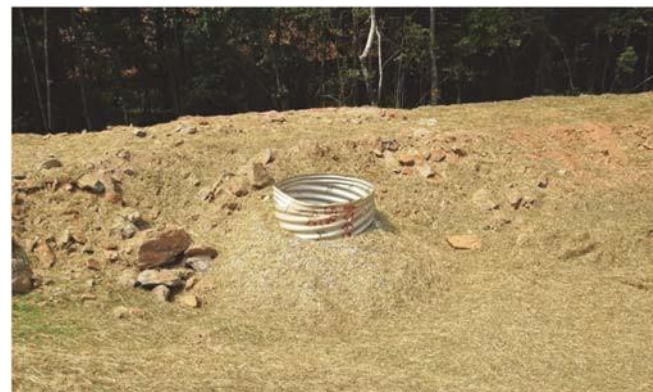
Inadequate rock around perforated riser. No trash rack.
