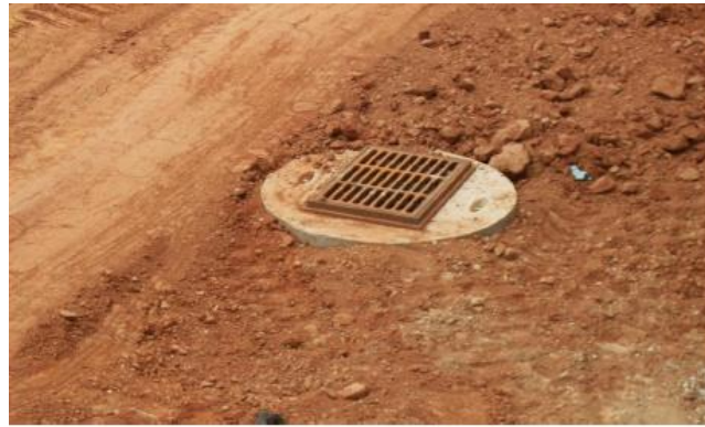
No attempt to protect inlet was made. Sediment rich runoff flowing directly into storm drain drop inlet.
