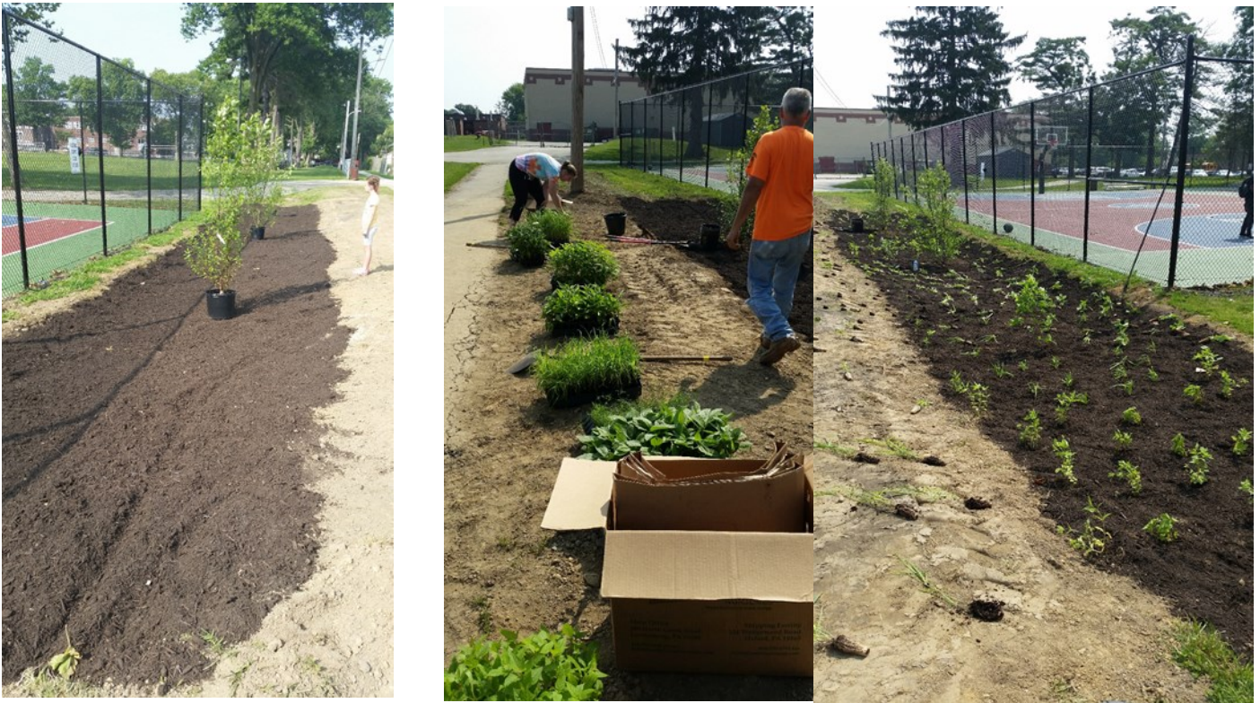
One of the Public Rain Gardens : This public rain garden shown during planting is in Sharon Hill in a borough park behind the Academy Park High School. Photo by Diana Andrejczak.
