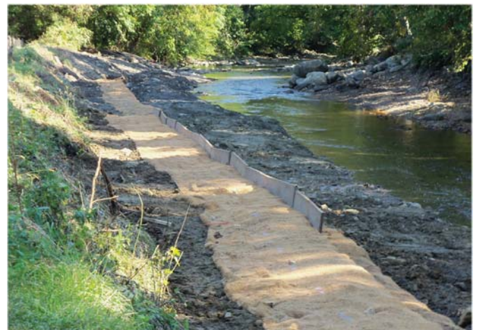
View downstream after Kent Park dam removal showing construction of the Vegetated Mechanically Stabilized Earth (coconut fiber matting filled with soil) and layered "terraced" to create a more natural bank slope
