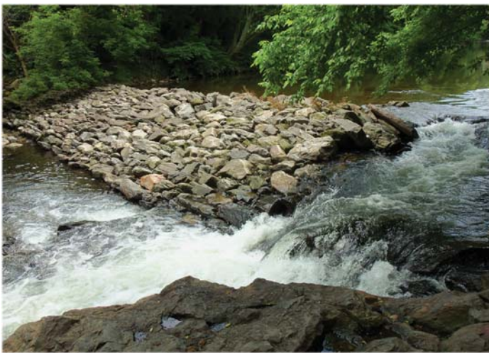
Kent Park Dam before removal. Note high water flow through breached area.
