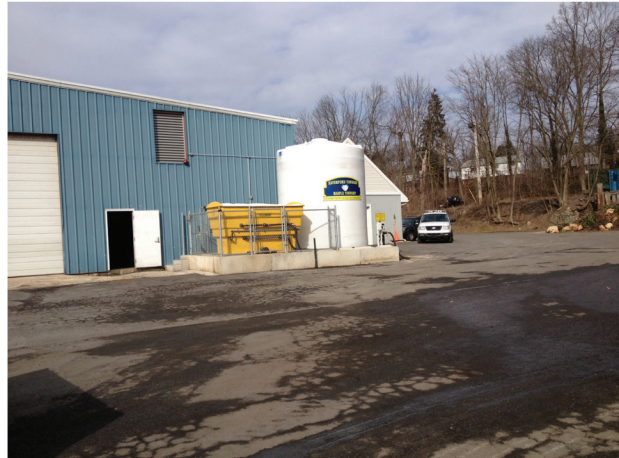
Haverford Township brine equipment
