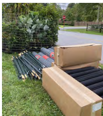
Metal stakes, caging and rigid trunk guards were used to protect the 140+ native trees and shrubs planted to manage stormwater at Gable Park.
