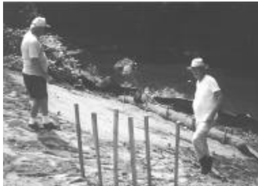
John Bowers (left) and Bill Frasch look over staked matting and BioLog at the stream stabilization project on Darby Creek in Darby Borough.
