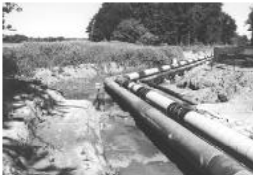
Sunoco oil spill site pipelines still exposed as work continues at the Refuge.
