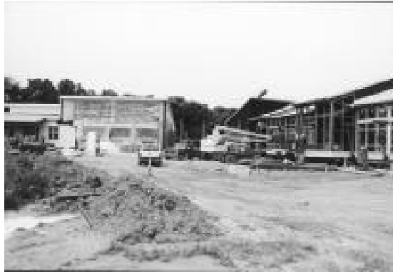
Work continues on construction of the Cusano Environmental Education Center at the Heinz Refuge.
